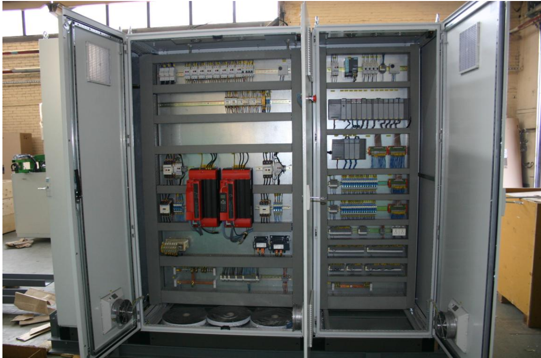
(1) 雙牽引機，PLC 電控箱。Double Puller, PLC Control Panel.
